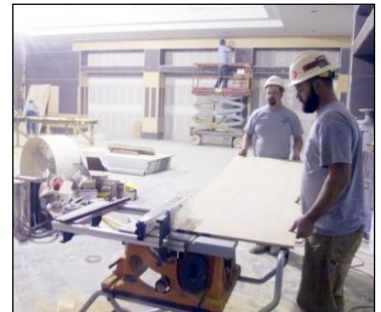
Construction of a beer and wine distribution center in Bay County is about 80 percent complete.
