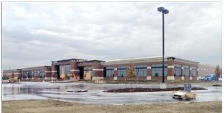
Construction is underway on a beer and wine distribution center, to be run by Fabiano Brothers Inc
